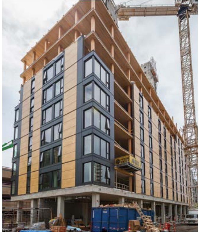
Brock Commons Phase 1 Student Residence is an innovative mass timber hybrid structure at the UBC. Image of construction progress July 2016. Photo Credit: KK Law
