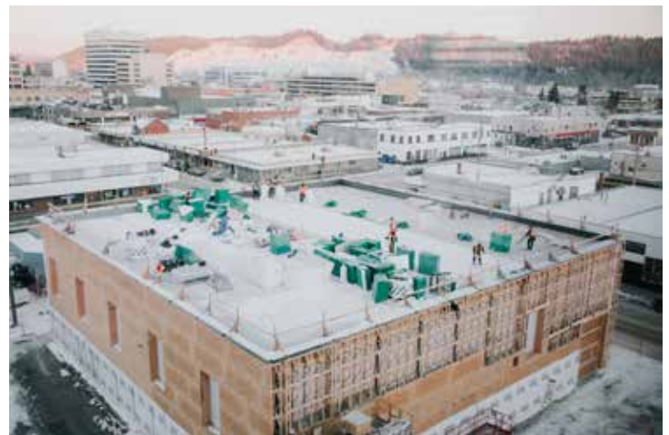
Construction of the WIRL in Prince George, B.C. Photos courtesy of UNBC
