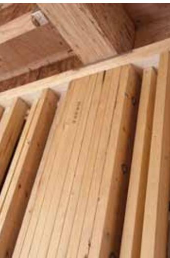
Top photo, seismic test conducted in Miki City, Japan in 2009. The prototype was built using BC forest products and incorporated construction techniques commonly used in Canada. Bottom photo, detail of column meeting ceiling rafter, Kamloops Library Square project.
